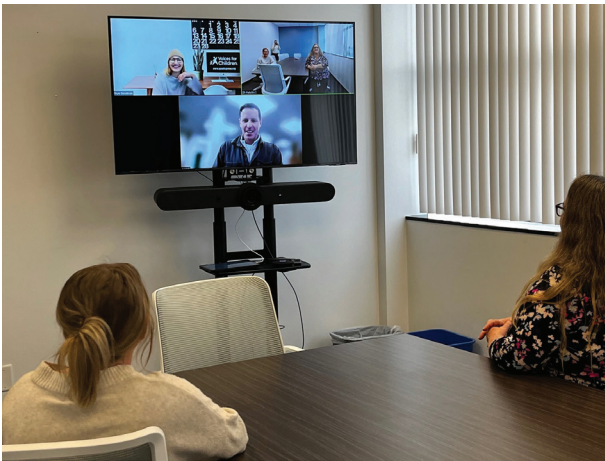
Above: Program Operations staff uses a newly installed video bar for effortless and effective virtual meetings.
